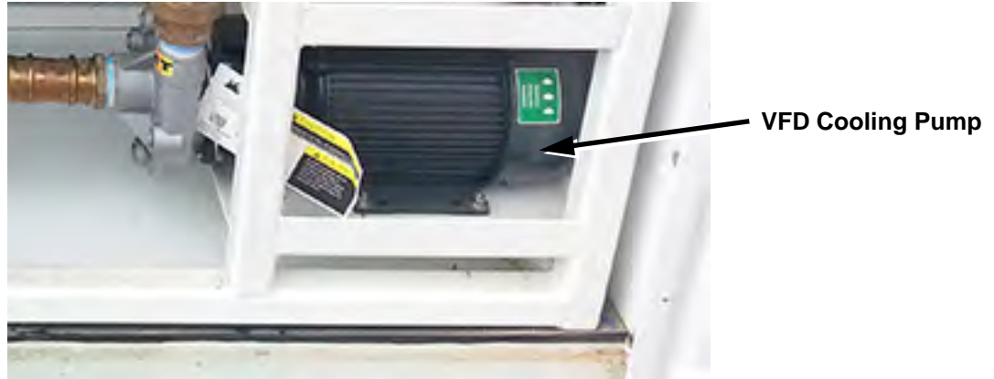
Figure 11: VFD Cooling Pump
