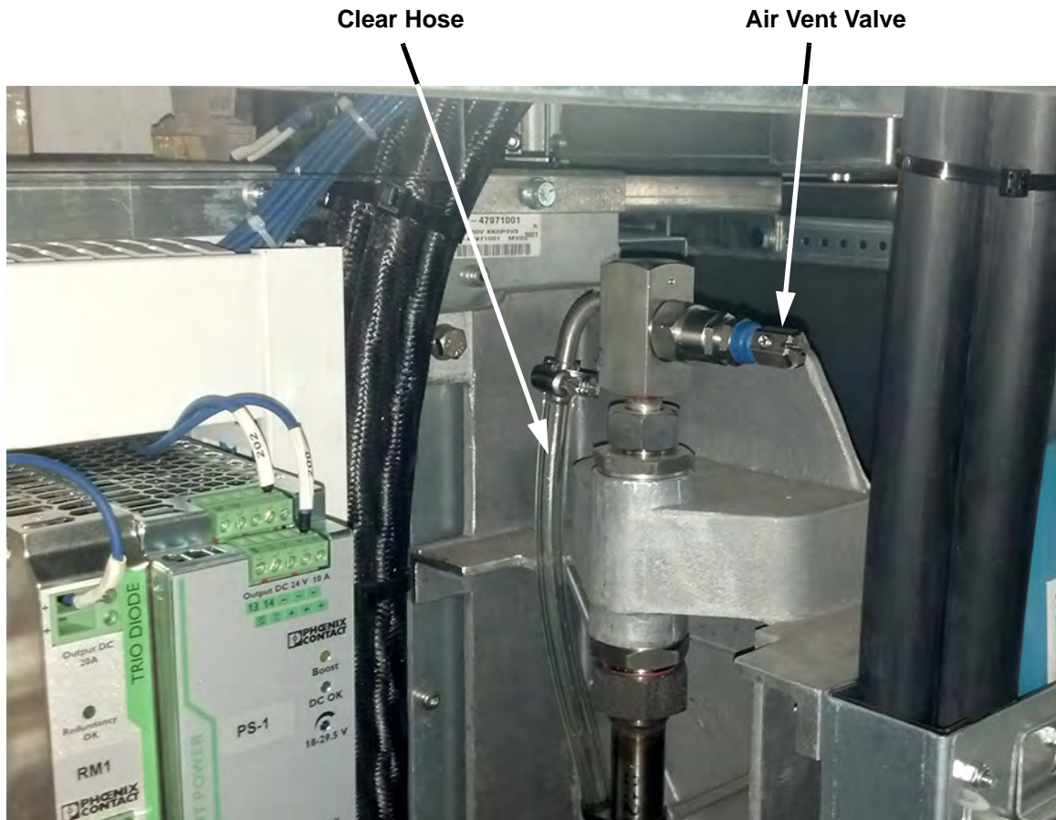
Figure 13: Clear Hose and Air Vent Valve in the VFD Delta Module
